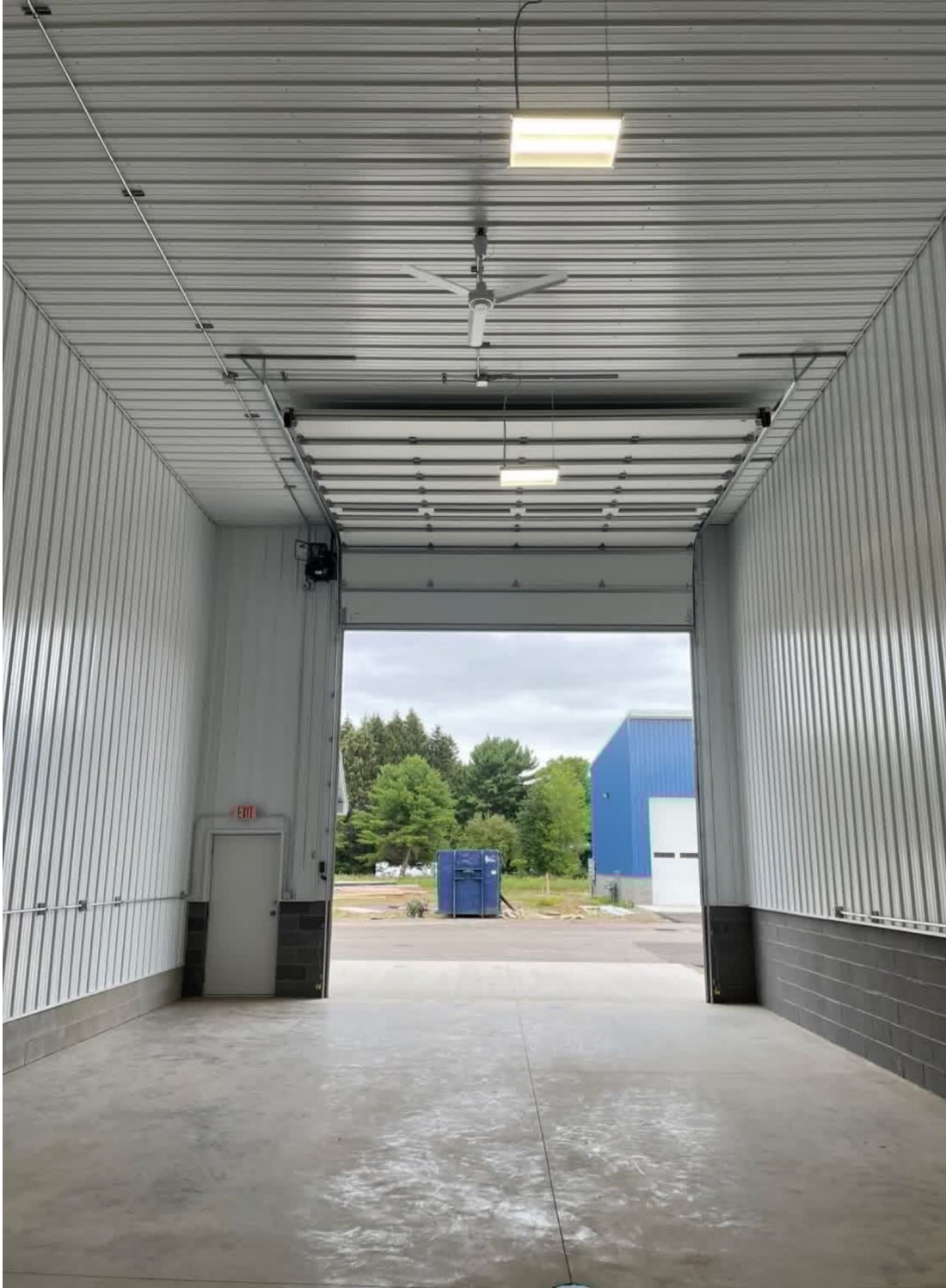
Interior lighting and steel liner panels
