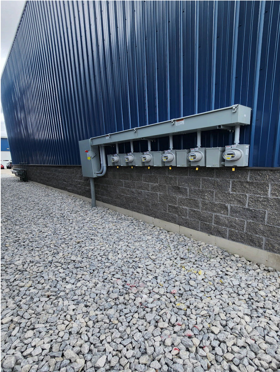
Individual utility service and metering
