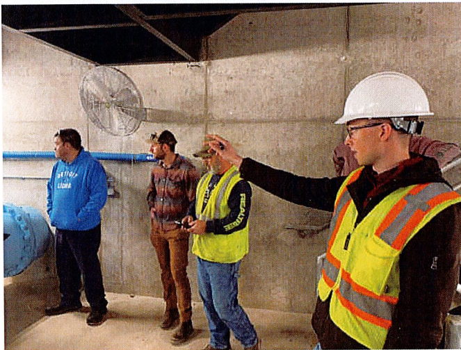
Will Theis of Prein&Newhof points out the features of the new high-flow West Randall Lift Station as our maintenance staff get training.
