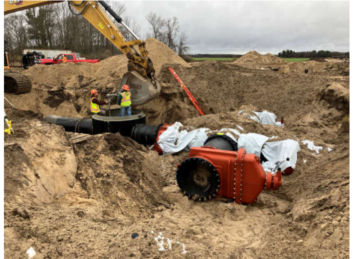
Workers install a manhole for an air release valve on the new section of irrigation main.
