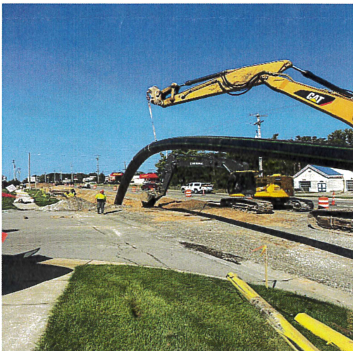
W Station Force Main Replacement: Installing fused HDPE pipe (22" O.D.) on Colby Road in Whitehall.
