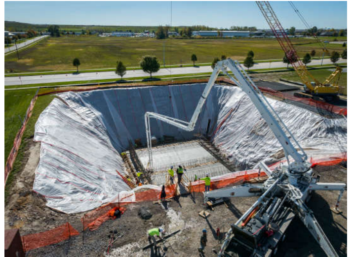
A drone's-eye view of the concrete pour for the base slab of the West Randall Lift Station. Photo courtesy of Prein&Newhof.
